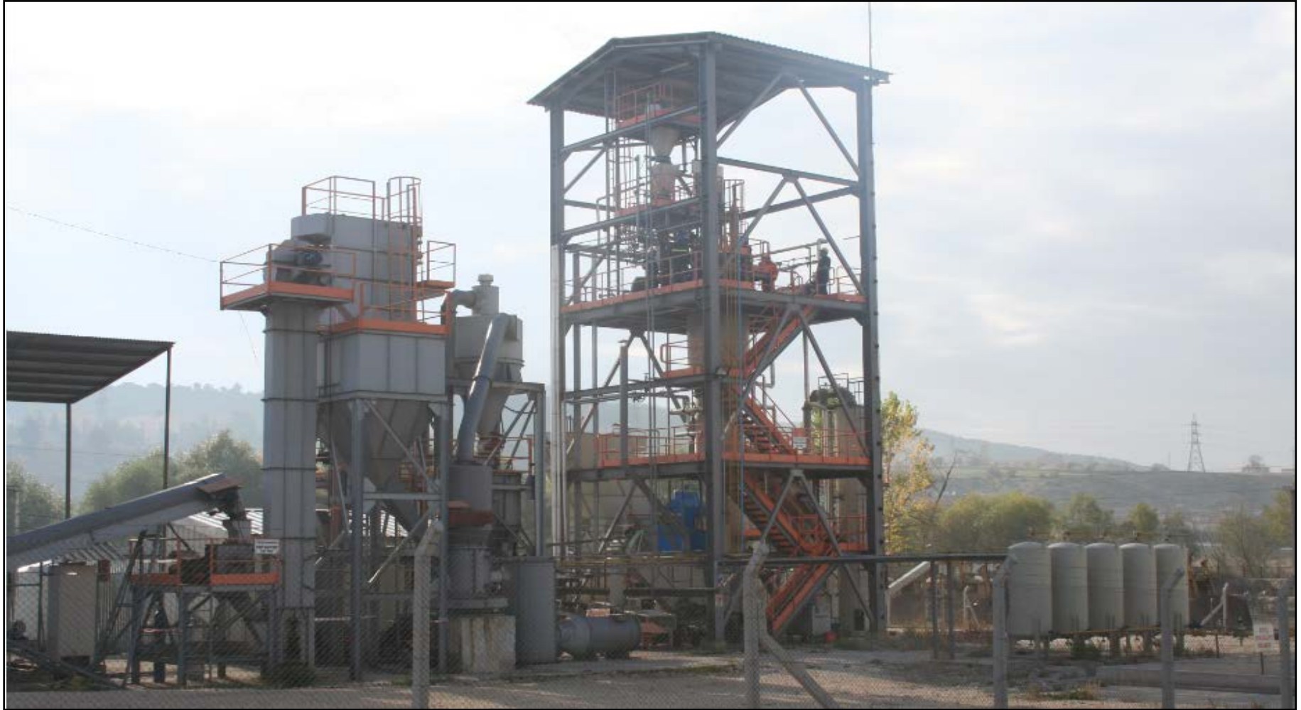
Entrained Flow Gasifier (250 kg/h)
